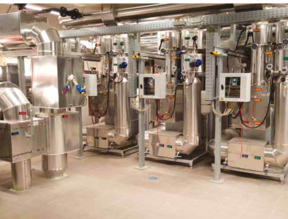
The primary side with the three transfer modules
