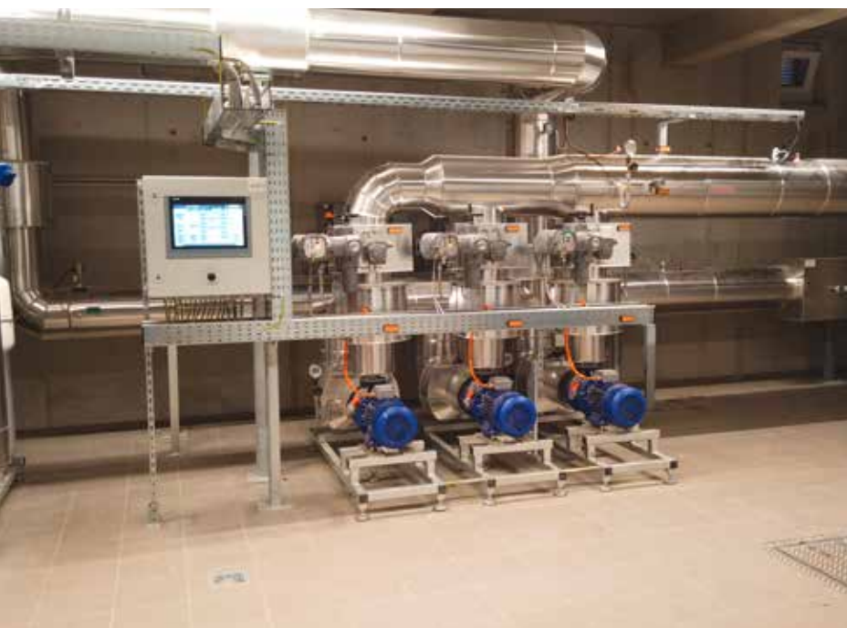
The secondary side with three pump modules to maintain the pressure
