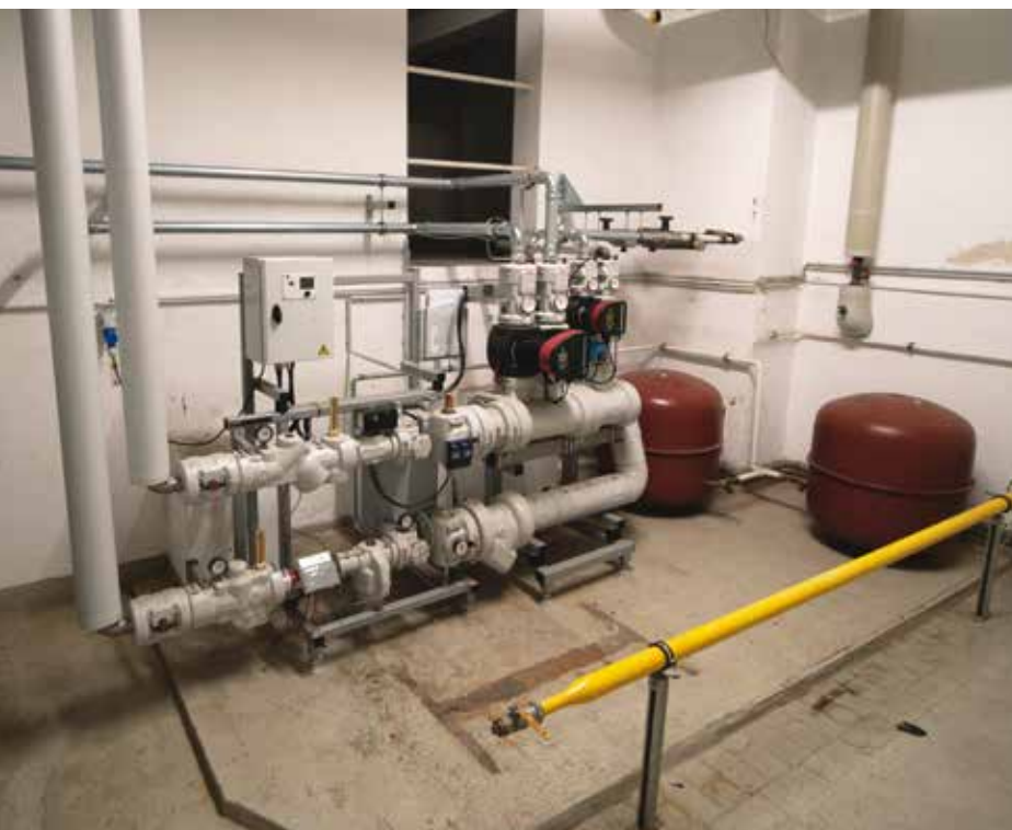
The ewers plant in the old coal cellar of the building
