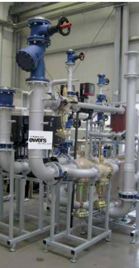
The ewers plant – Modular design 3 MW consisting of full load module 2.5 MW and partial load module 0.5 MW
