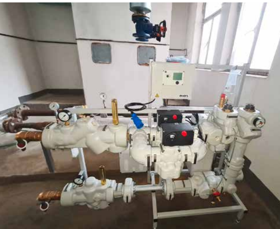
Station for district heating transfer
